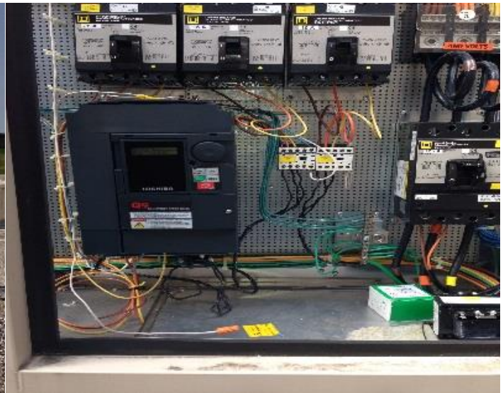
VFD on control board inside RTU
