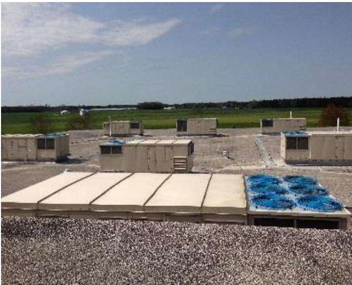
9 Roof Top Units had Toshiba VFD's installed
